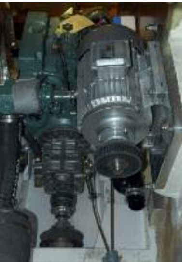
Diesel electric and hybrid installation.
