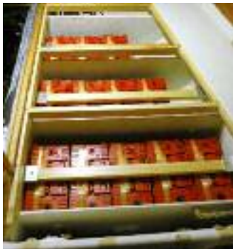
144 v battery bank
